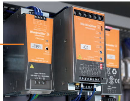
ESG: All-purpose equipment identification - simple labelling of markers for quick identification of components
